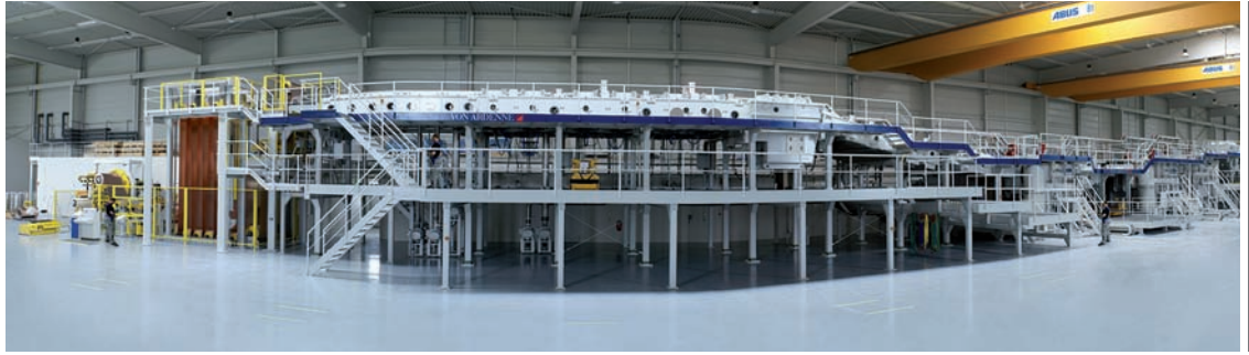
The vacuum coating facility in Bernburg is one of the most modern in the world.
